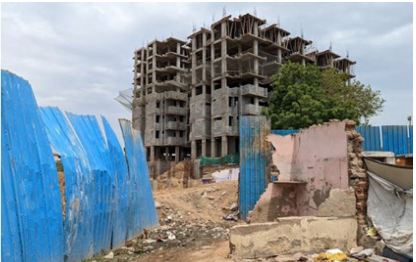
Apartments under construction on the site of demolished houses in Rama Pir No Tekro, Credits: Rahethan Adhikar Manch, Gujarat
