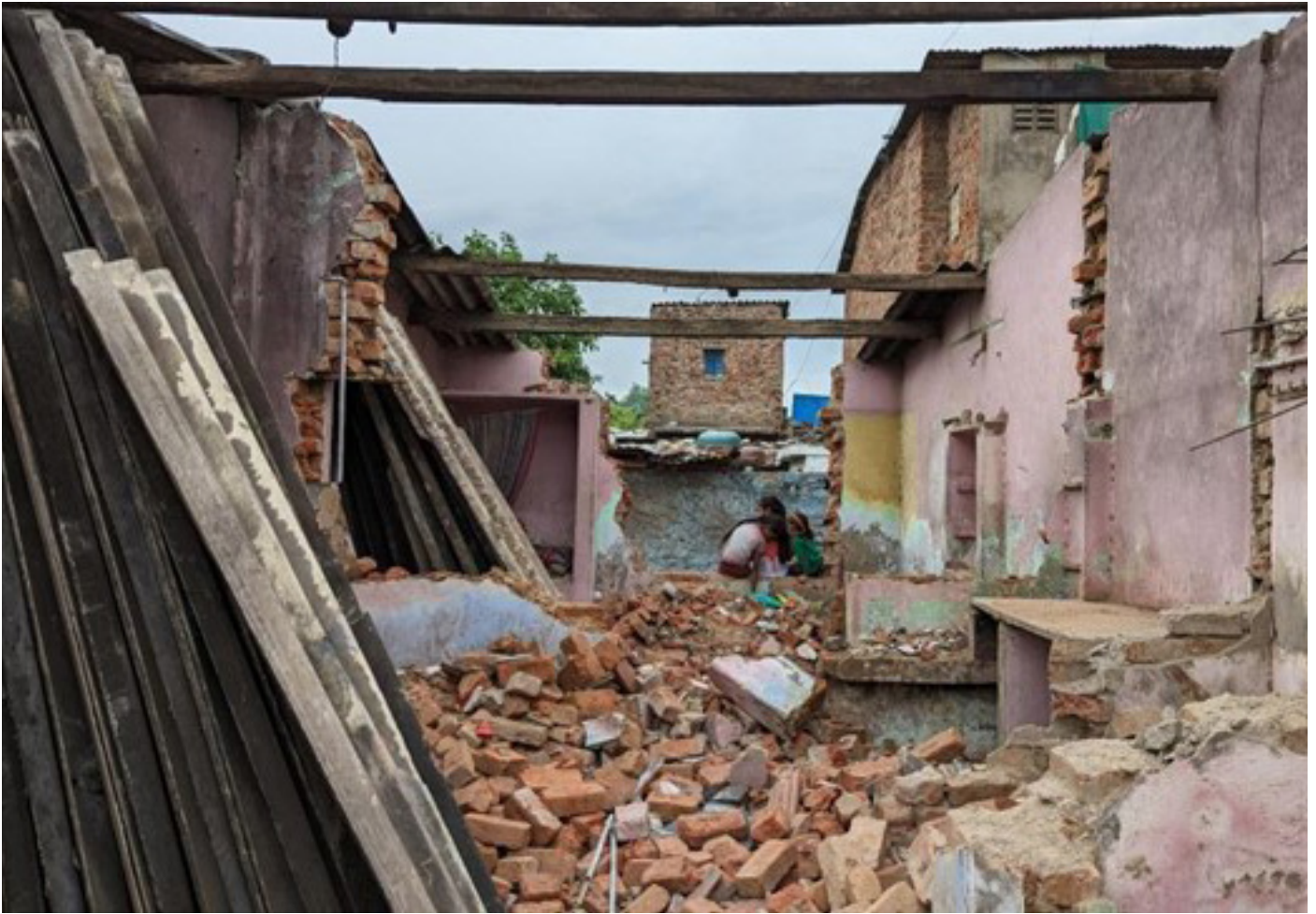
Partially demolished homes in Rama Pir No Tekro, Credits: Rahethan Adhikar Manch, Gujarat
